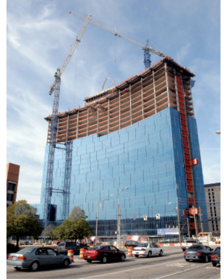
The convention center connects to the new $450 JW Marriott, seen here under construction in early 2010, via climate-controlled walkways.
