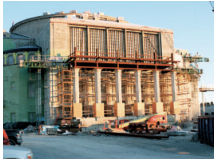
Currently under construction, the Regional Performing Arts Center will open this year.
